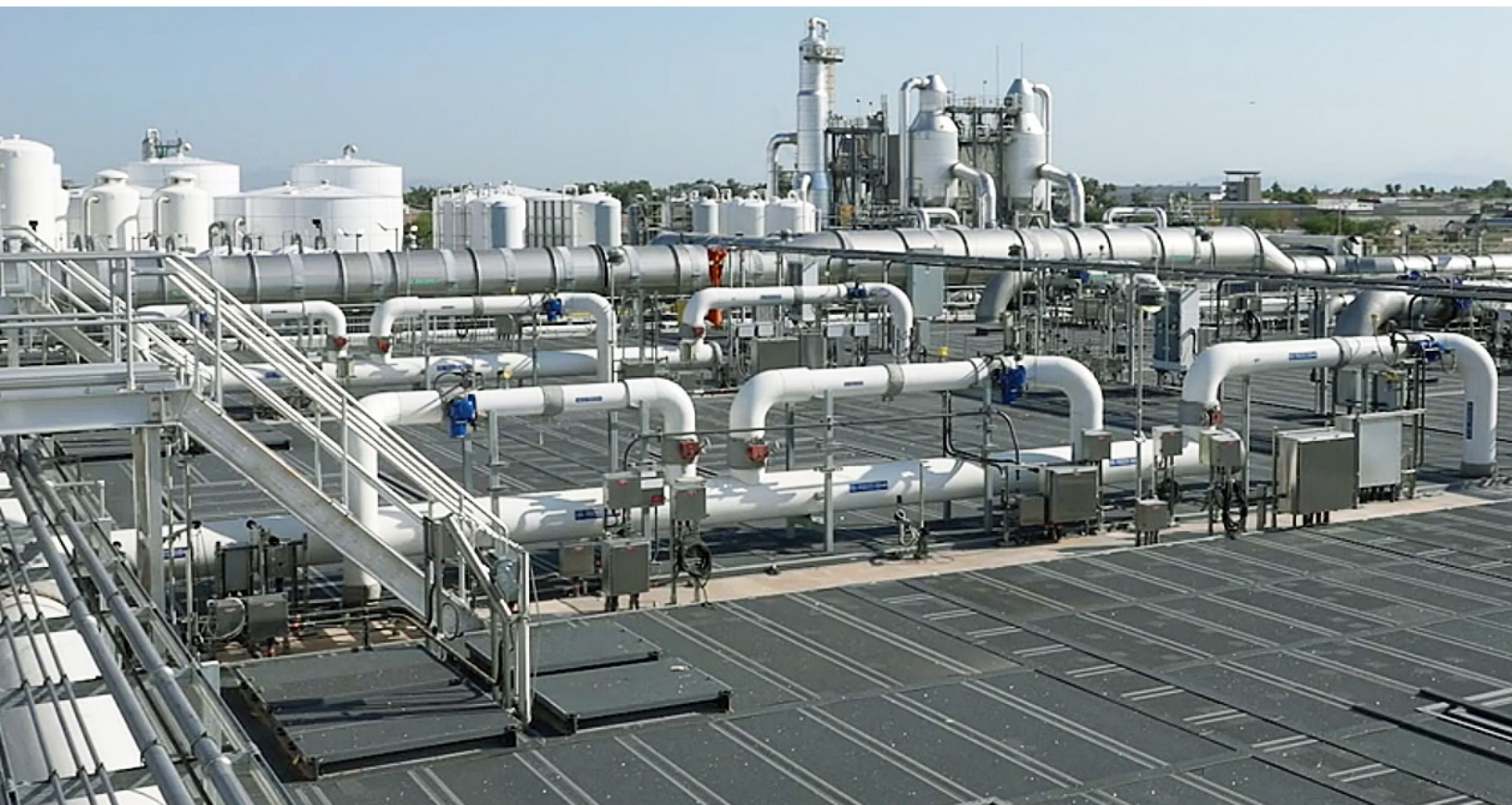
WATR treatment facility in Ocotillo
