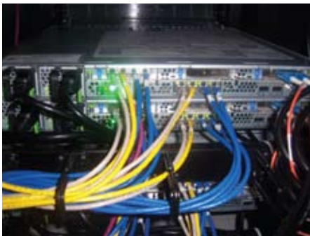
Figure 1. Configuration of the server wiring when using eight 1GbE connections.
