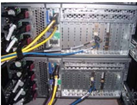
Figure 2. Configuration of the server wiring when two 10G connections replace eight 1GbE connections.
